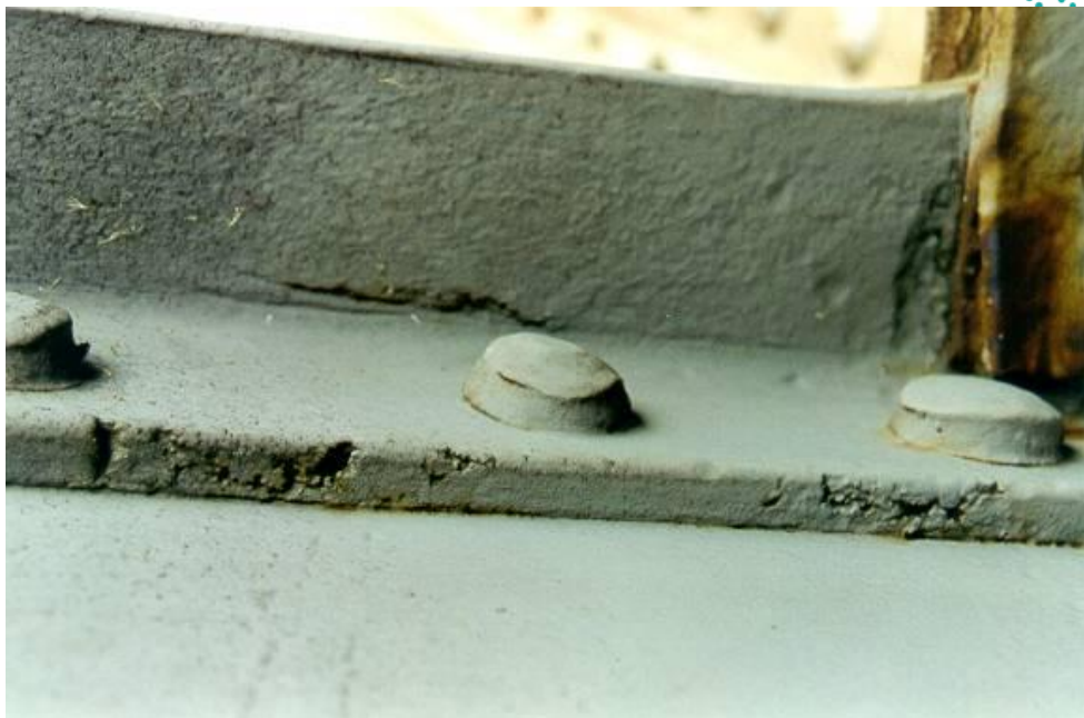
Figure 14 - Poor quality wrought iron can often be identified by defects on the edges of the rolled section. Edges often show the straight outline of laminations and delaminations
