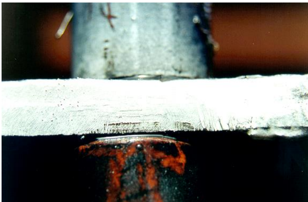
Figure 17 - After application of mpi laminations show clearly, positively identifying wrought iron
